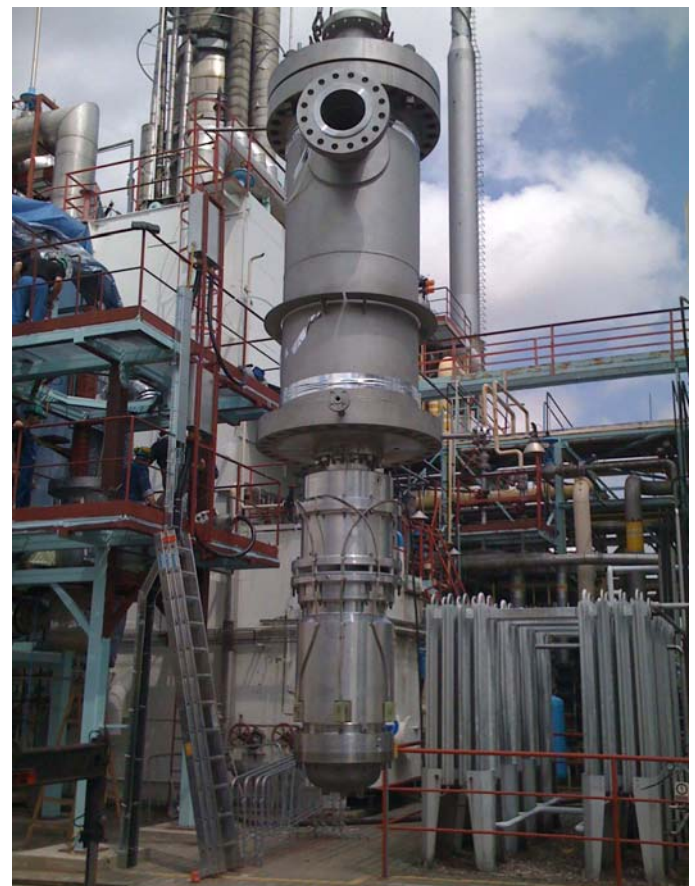
Figure 18: Installation of the Tandem Configuration in Poland in 2009
